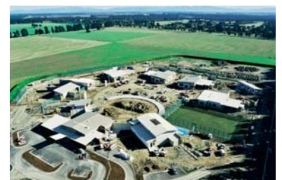
Client: Child, Youth and Family Architecture and Building Engineering Services: Stephenson & Turner
