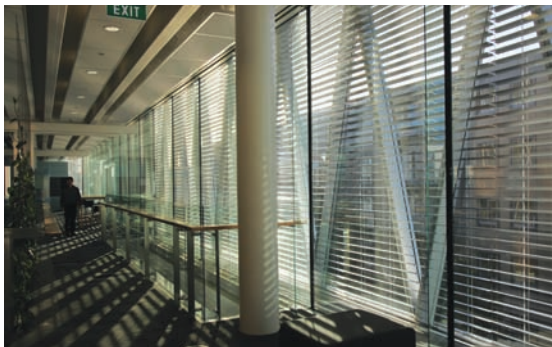
Automated blinds in twin cavity
